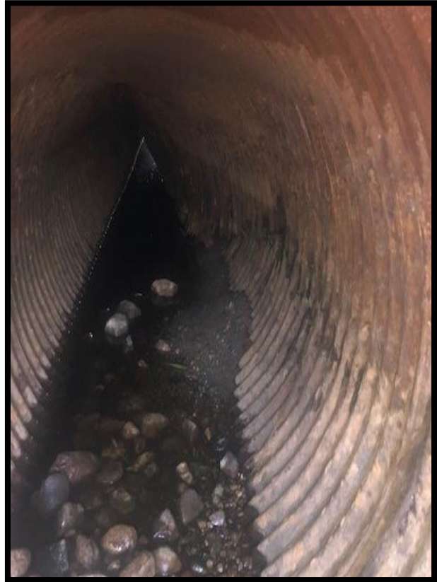
Take photos of inside of culvert prior to excavation to determine condition
