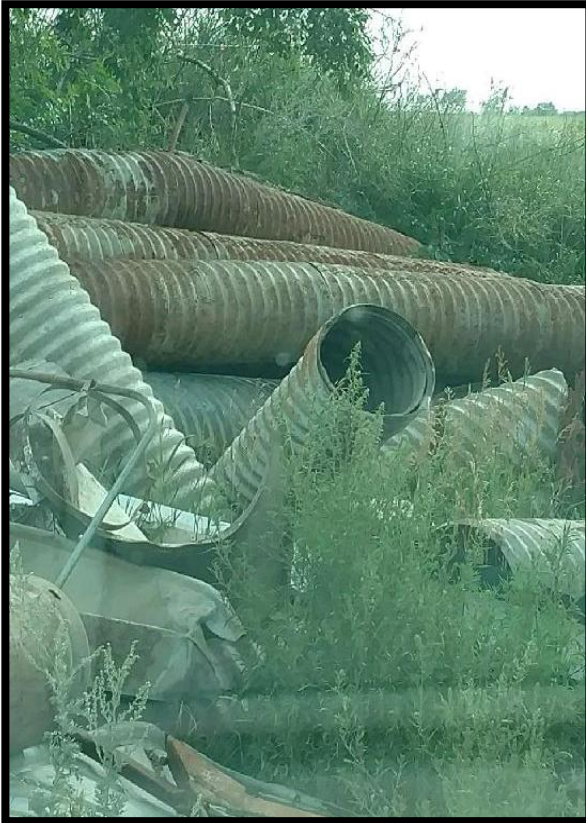
Take photos of damaged culverts to identify condition if excavated
