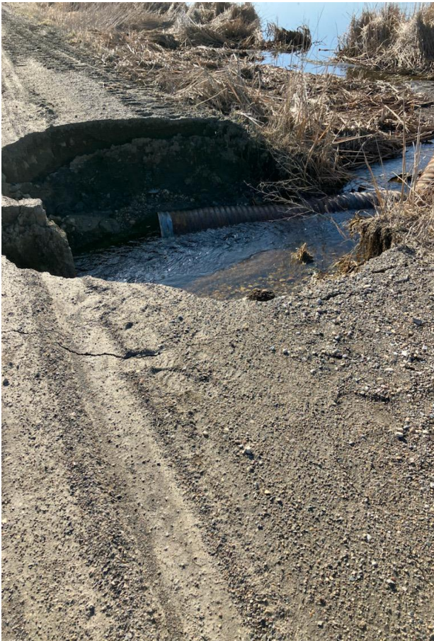
Photo captures erosion and separated culvert (Good)
