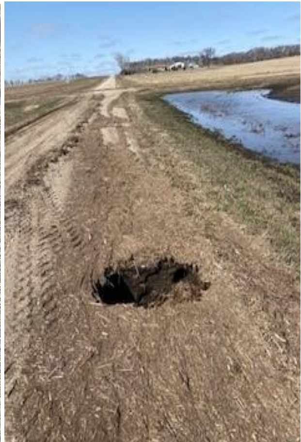
Photo identifies hole in road. Damages Typical of a rusted culvert or animal damage (Poor and not eligible without additional photographic evidence – Have contractor take pictures of when repairing...)
