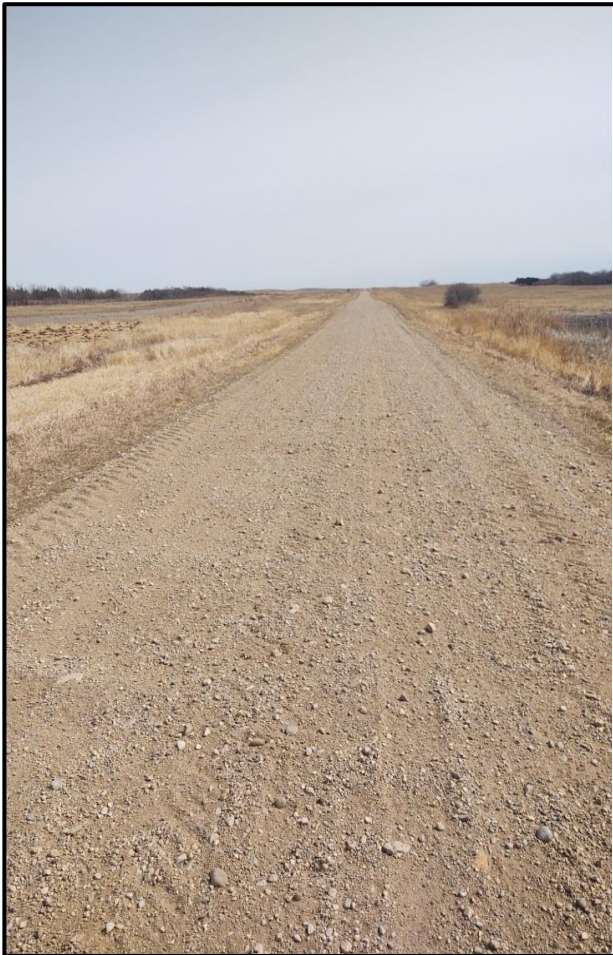
Photo does not show gravel wash (Poor)
