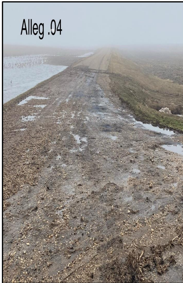
Photo does show gravel wash (Good)
