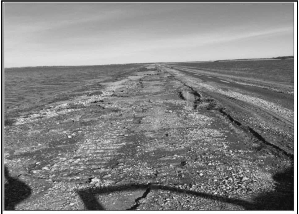
Example of a road that was completely submerged in water for an extended time. Debris needs to be cleaned up and re-graveled. (credit: North Dakota Department of Emergency Services)
